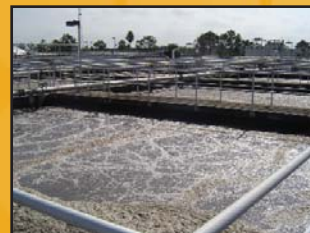
Aeration bays at a wastewater treatment plant
